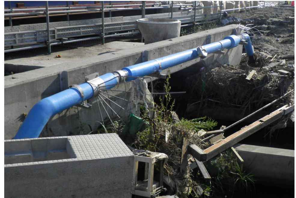
Pipe bridge, completely broken air valve
