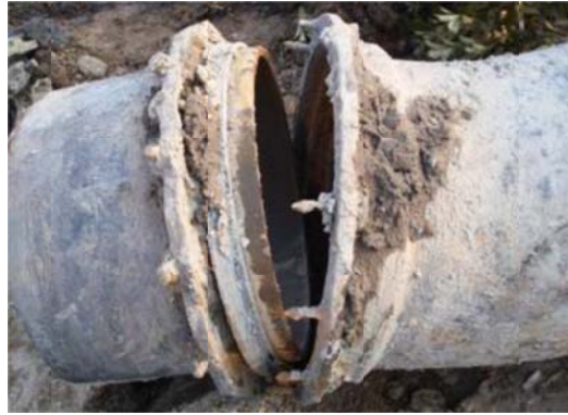
Figure 3. Joint pullout in a ductile iron pipe, [5]
