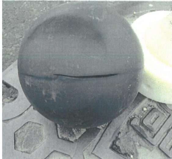
Photo 2. Damaged float valve body
