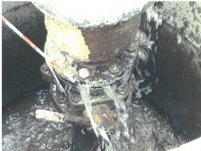
Photo 3. Leakage from flange joint
