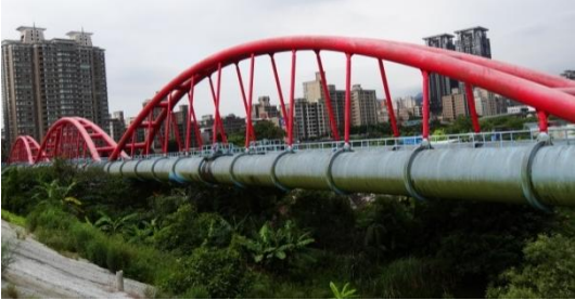
Hsintien arch water pipe bridge
