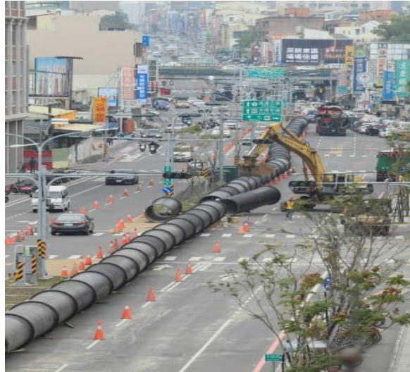
Fig.3 1,350 mm emergency temporary transmission pipe on the ground
