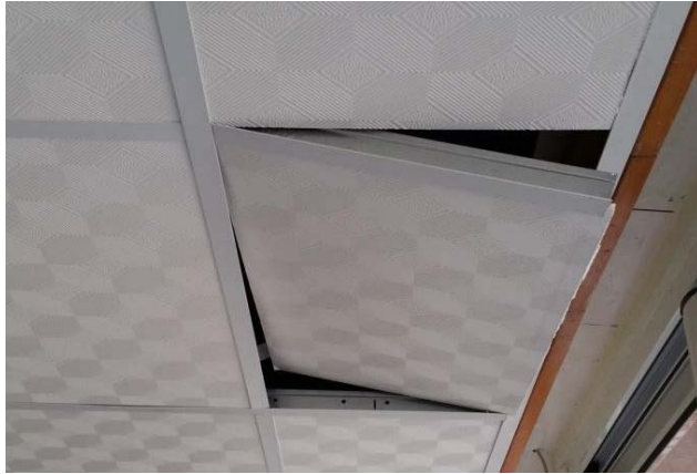
Seismic-R Ceiling Grid/ No Brace
