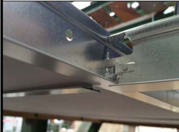
Damaged latches of cross tee
