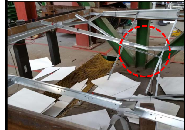
Damaged main grid
