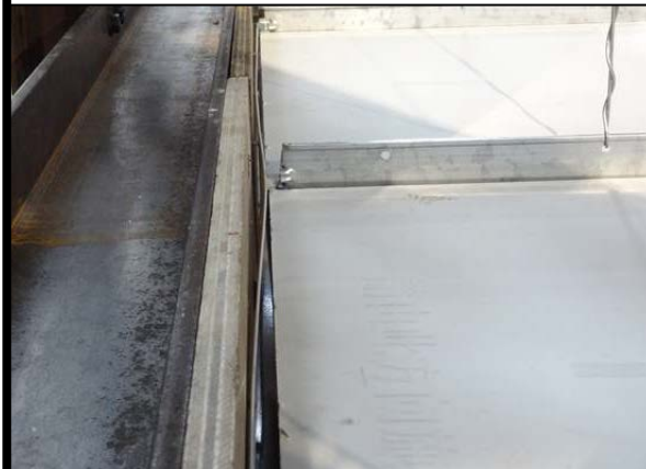
Damaged wall moldings
