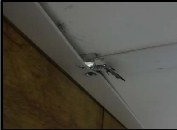
Damaged perimeter connection
