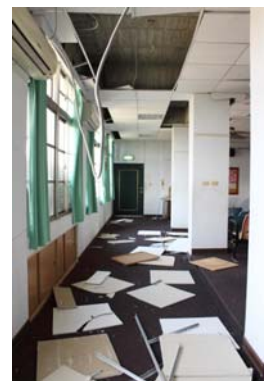
(b) 輕鋼架天花板掉落
