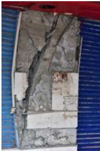
(c)一樓柱剪力破壞
