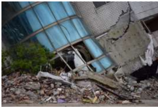
(e)邊柱破壞
