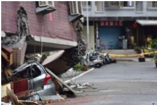
(c)一樓柱及梁柱接頭破壞
