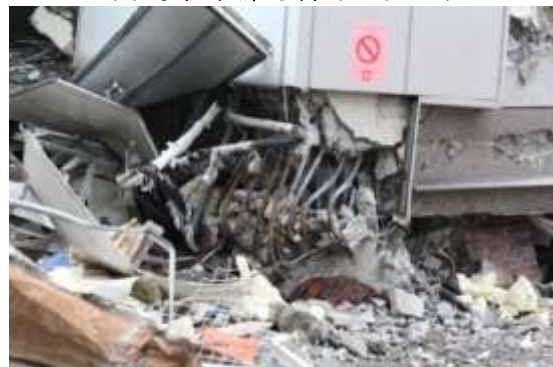
(f)角柱破壞
