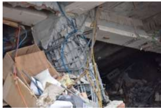
(f)內柱破壞
